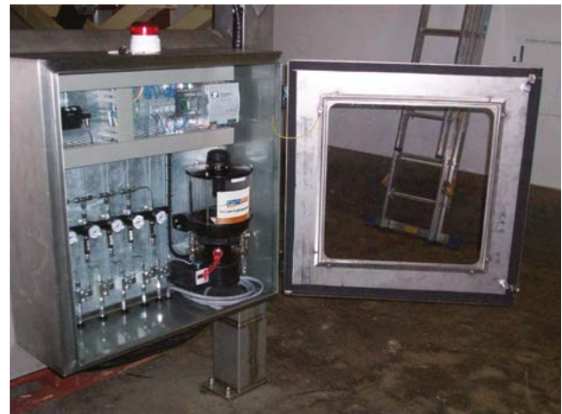
Figure 3: There are many types of centralised lubrication systems for an entire plant. The most common type is an oil circulation system.
