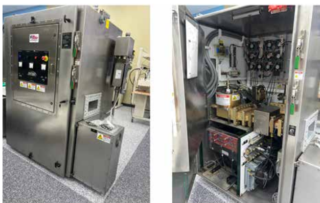
Figure 12: A 75 KW Microwave Transmitter with 5ft x 4ft Footprint Showing Magnetron, Circulator and Waveguide opening on the outside 13
